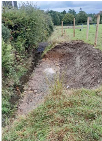
Photo 13: Slurry trap which can be closed off in the event of an accidental spill.
