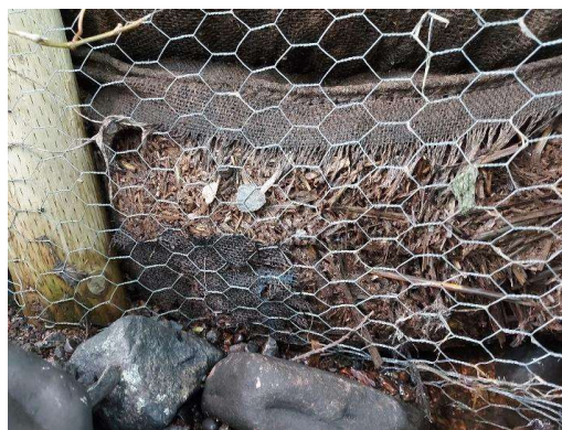
Evidence of log deterioration
