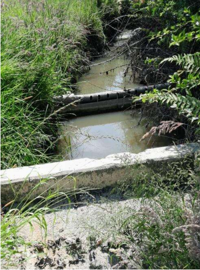
Photo 11: Check dams and pipes carrying water off to a parallel swale when levels get higher.
