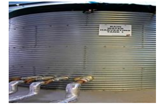
Water header tank (30m 3 )
